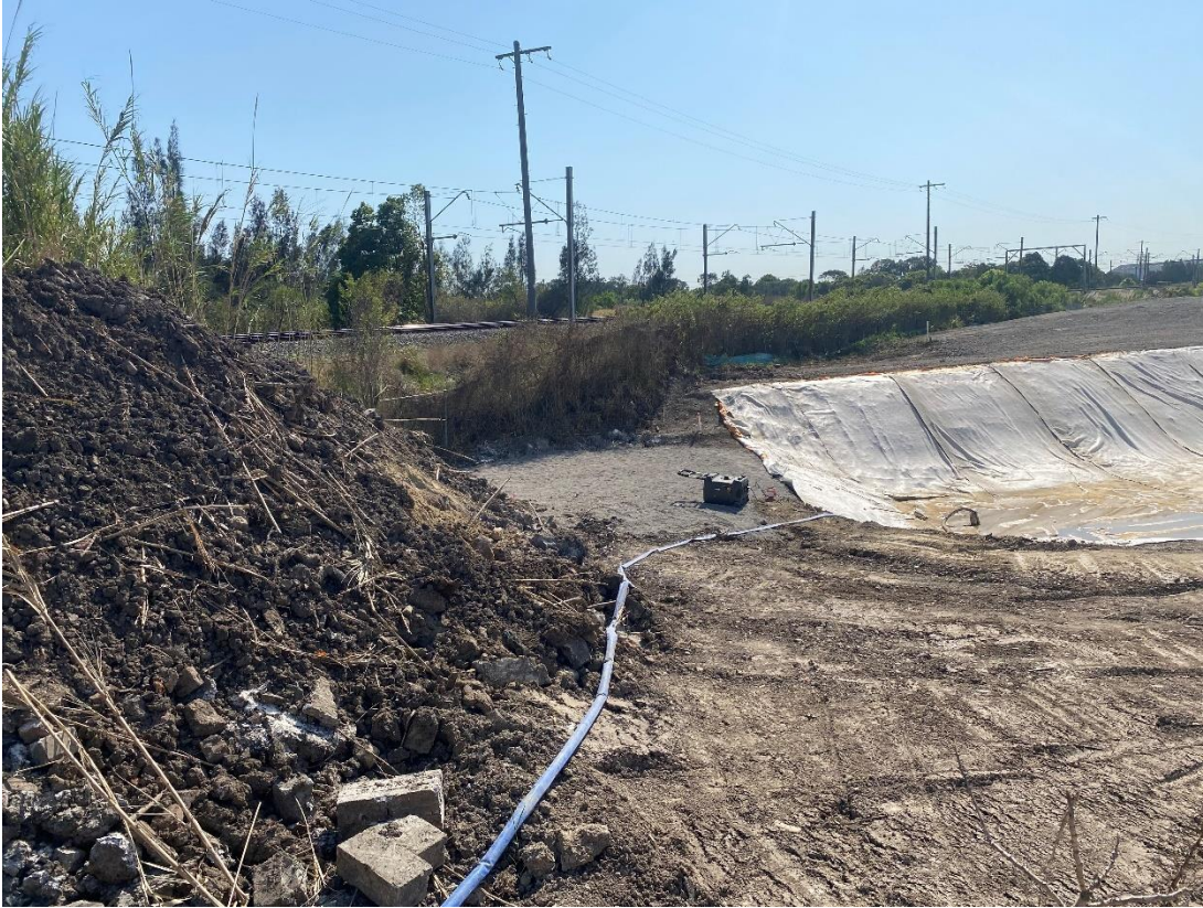
Photo 7 At the time of Day 1 of the site inspection water was being pumped to Sediment Dam 2 from Sediment Dam 1 to finalise its construction. Auditor advises drain needs minor reshaping to minimise risk of uncontrolled discharge off site.
