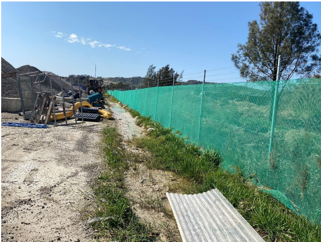
Photo 12 Southern drainage line is mostly vegetated.
